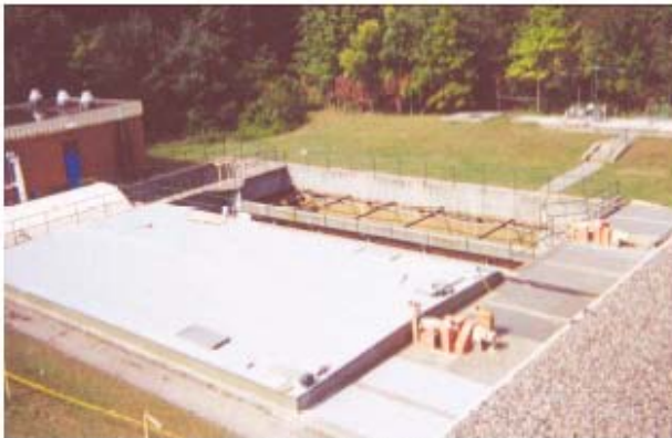
Odor control covers at a wastewater treatment plant in Smithfield, Rhode Island, will withstand the corrosive environment to provide years of trouble-free service.
